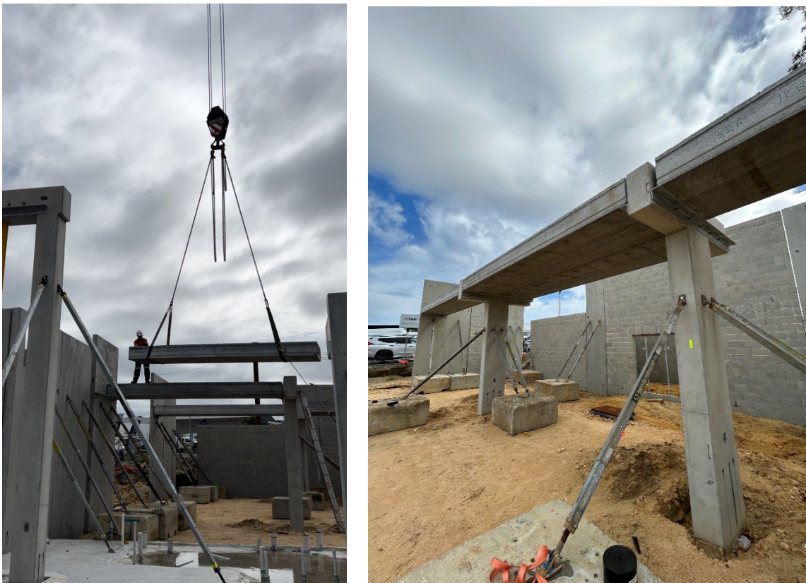
Figure 5 & 6. CVB Installation at Audi Centre Myaree
